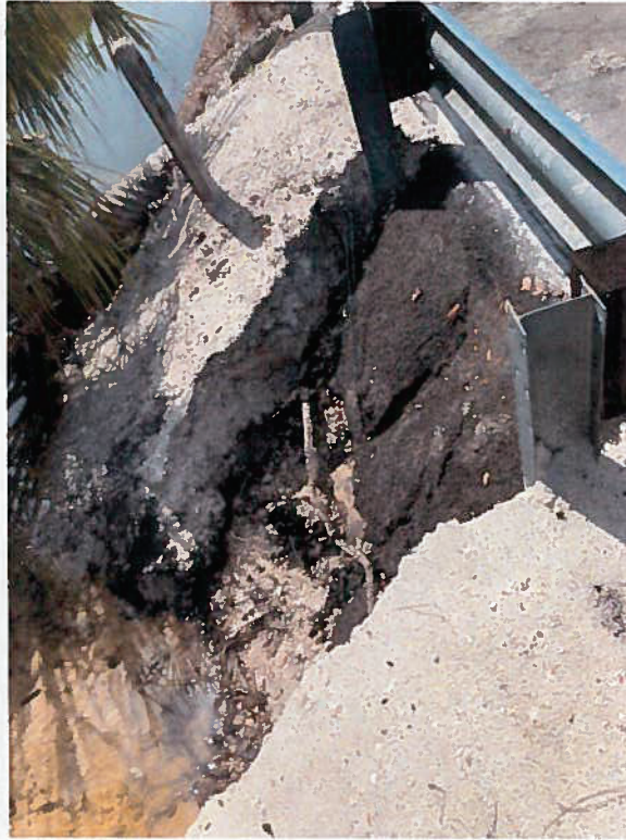
Figure 25 – Area of continued erosion
