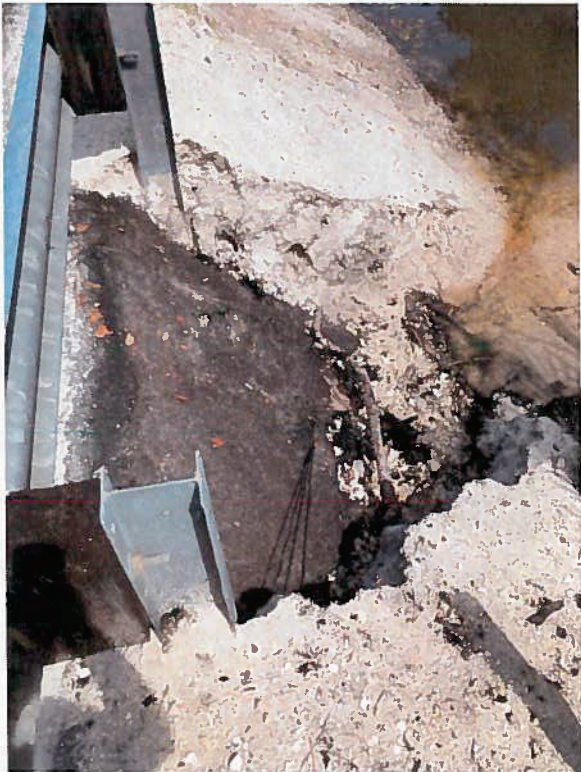
Figure 28 – Area of recent erosion
