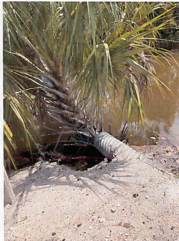
Figure 26 – Tree growing out of canal bank
