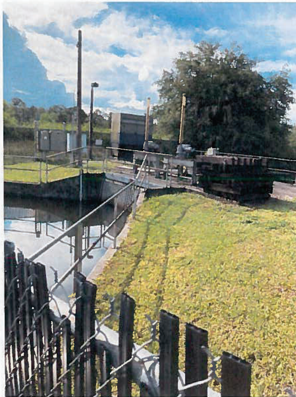
Figure 42 – Back-up generator at Control Structure No. 1
