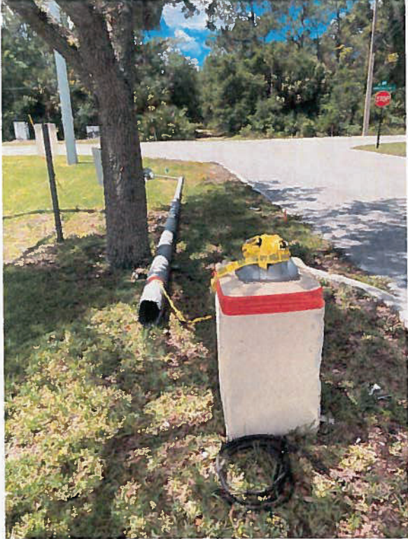
Figure 49 – Damaged light pole near intersection of Innovation Drive and Endeavor Drive
