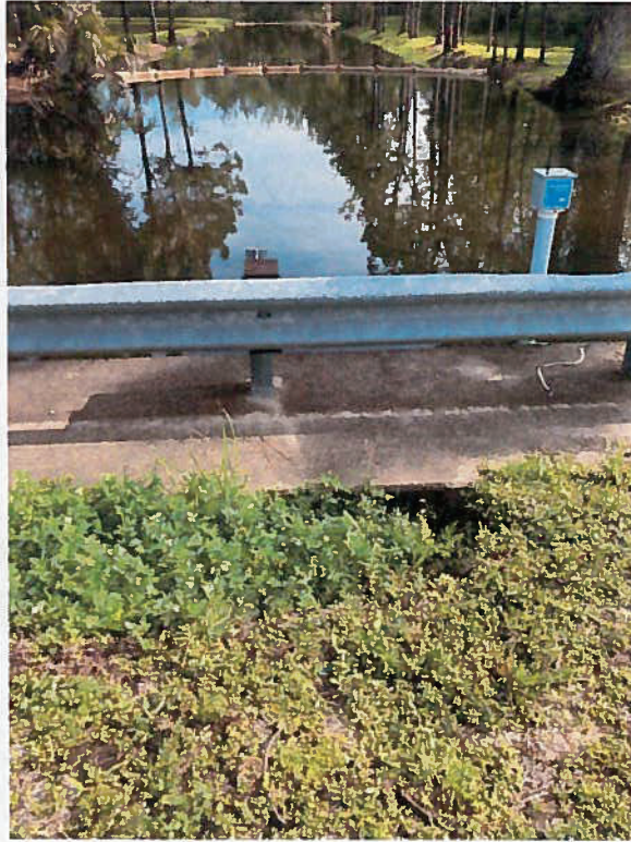
Figure 2 – Closer view of erosion behind headwall
