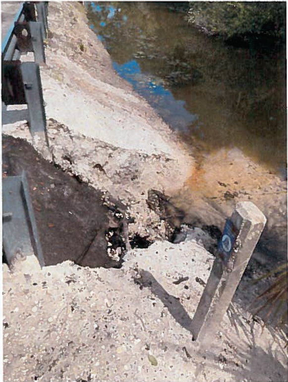
Figure 27 – Same area of recent erosion
