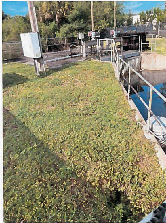
Figure 38 – Electrical panel at Control Structure No. 1
