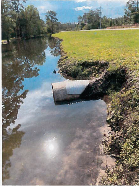
Figure 14 – Erosion of canal bank on north end of slip-lined culvert under Innovation Drive
