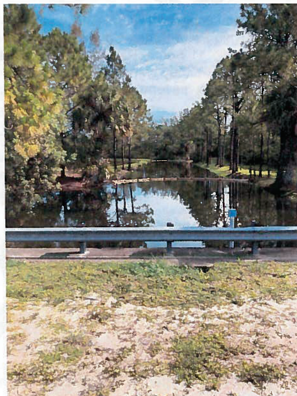
Figure 1 – Looking north at canal on east side of stormwater tract, upstream of pump station. Note erosion at backside of the top of headwall.
