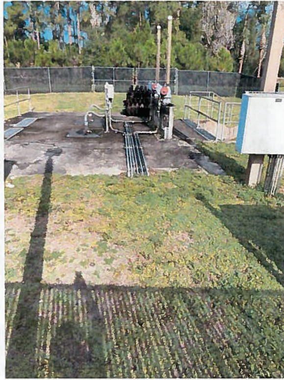
Figure 37 – Gate actuators at Control Structure No. 1
